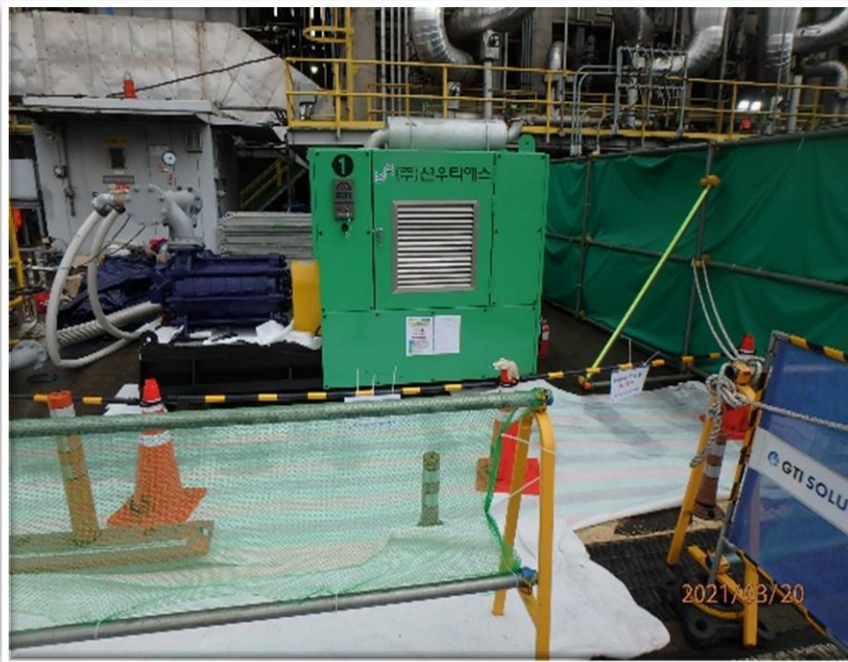
Decoking Water Pump
